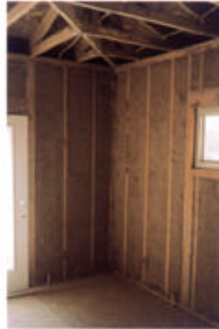
The new generation of cellulose is the foundation of the energy efficient home. Pictured here are master bedroom walls insulated with wet-blown cellulose before sheetrocking.
